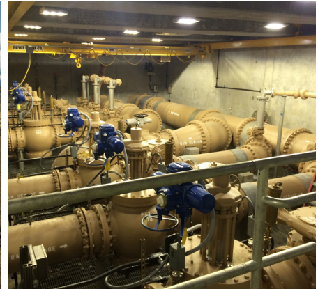
Peachtree Creek Relief Storage & Pump Station
