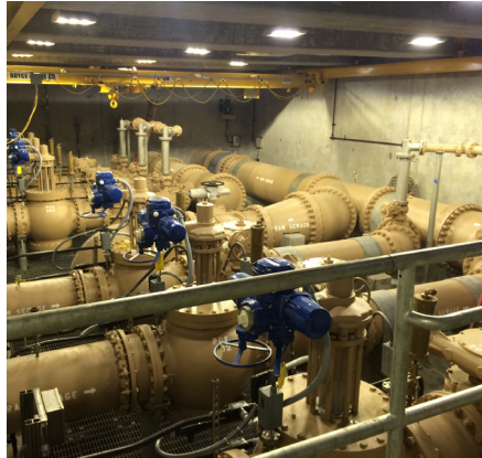
Peachtree Creek Storage and Pumping Station
