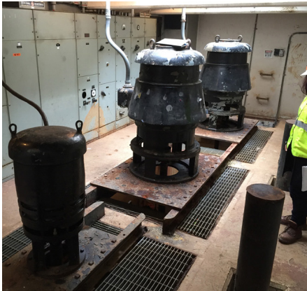
Emergency Generators, DC Water and Sewer
