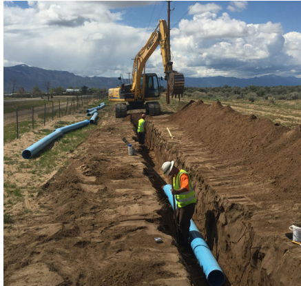
Sierra Army Depot (SIAD) Potable Water Well
