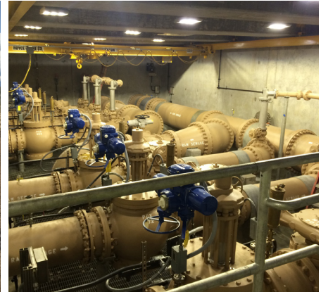
Peachtree Creek Relief Storage & Pump Station
